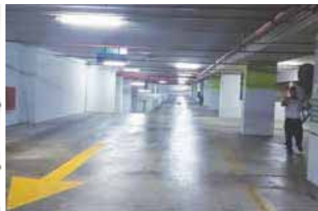
Figure 28: Installed energy efficient LED lighting
